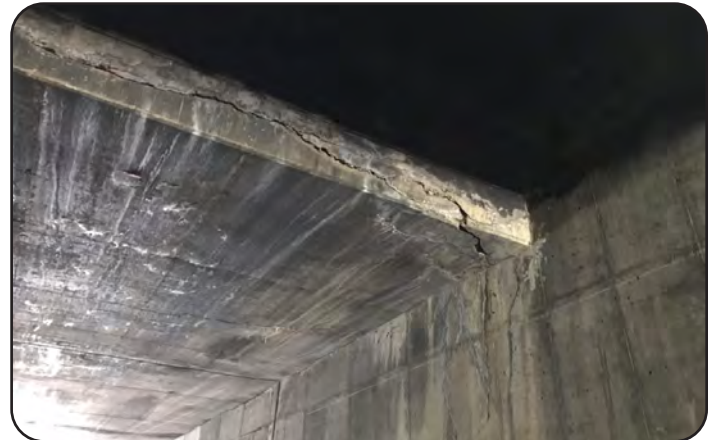
Image 8. Severe Cracking on I-70 over Forest Service Rd (F-13-S_Minor)
