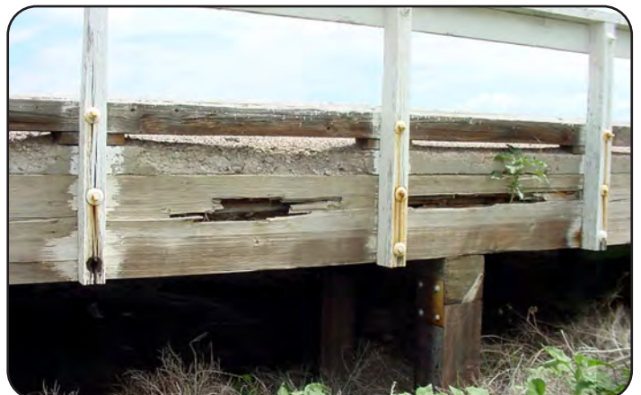
Image 4. Rotting Girder on US 36 ML over Draw (F-19-E)
