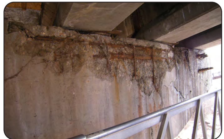
Image 12. Severe Abutment Deterioration on I-270 EBND over S. Platte River (E-17-IE)
