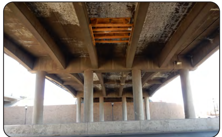
Image 2. Severe Deck Deterioration on I-70 WBND over West 32nd (E-16-HF)
